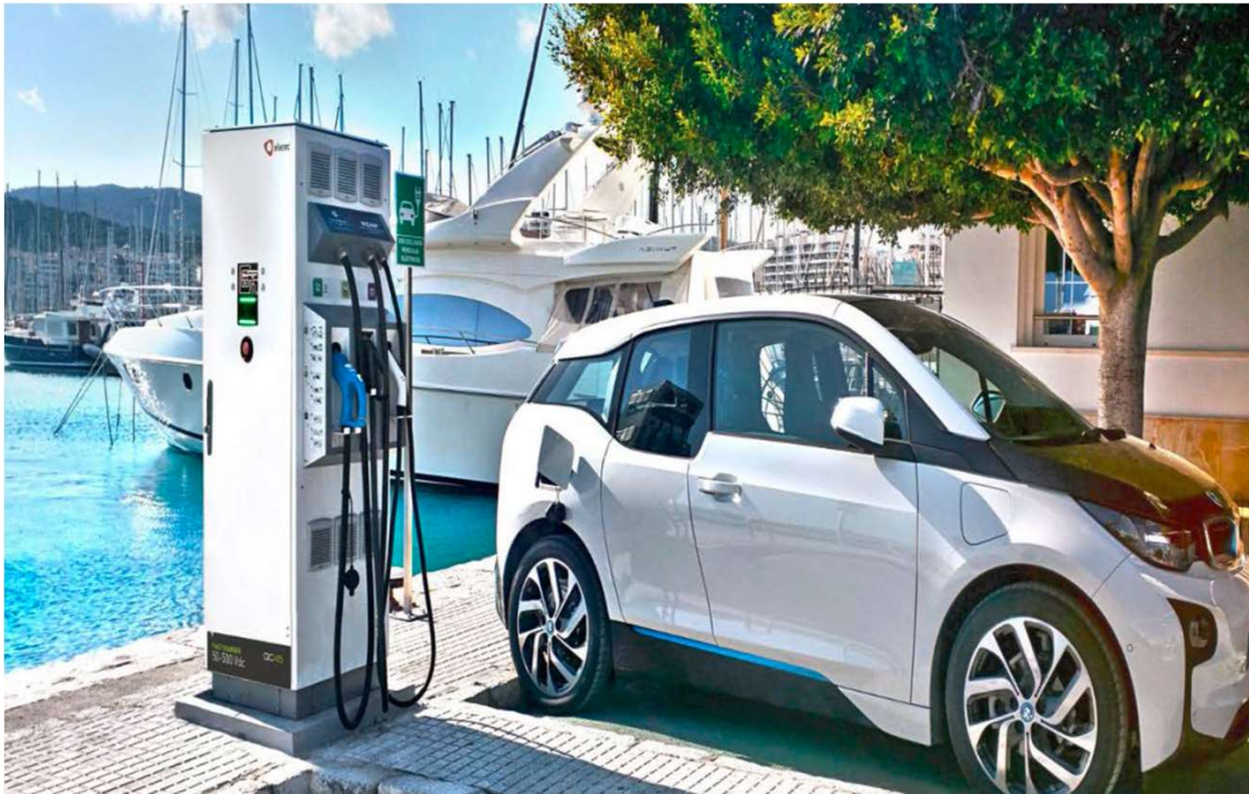
E-filling station with 3 ports, covers all electric vehicles currently available on the market.
